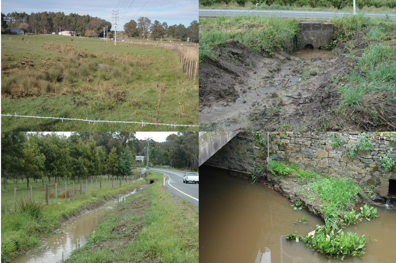
Figure 5. Examples of burrowing crayfish potential habitat, including low lying areas with a shallow watertable, modified areas such as drains and culverts, and small remnants of habitat in highly modified areas.
